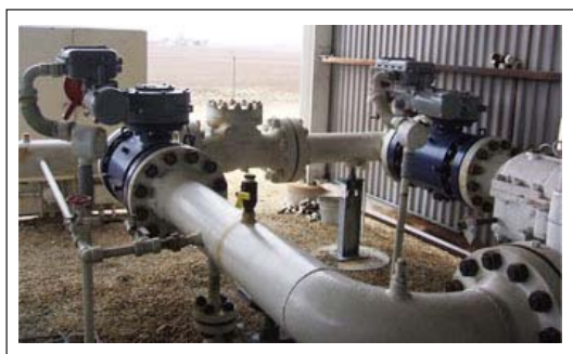
Crude Oil Pumping Station Pig Launcher/Receiver
