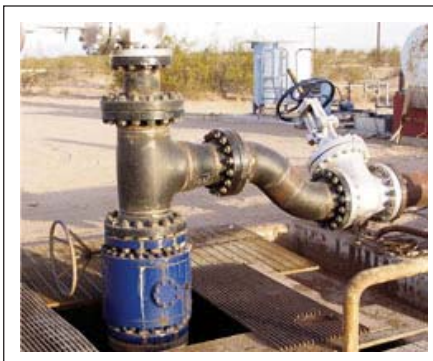
Master Valve Geothermal Brine
