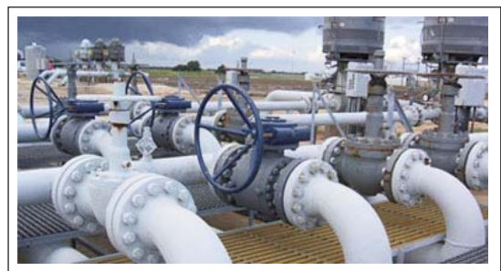
Salt Dome Brine & Gas Pumping Station
